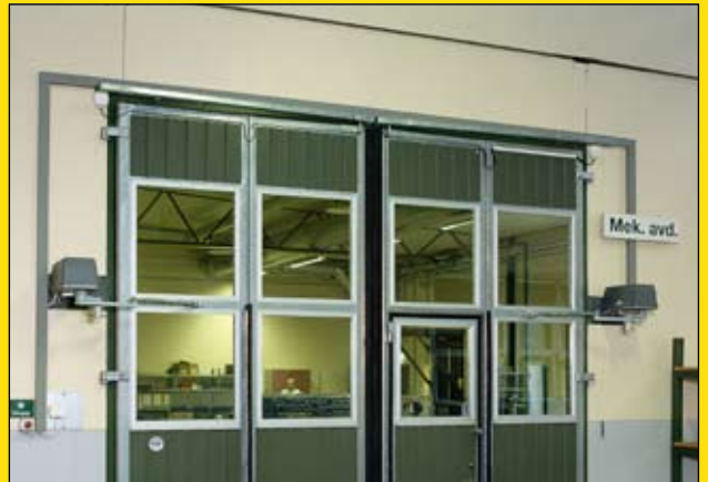
MT installed on a folding door
